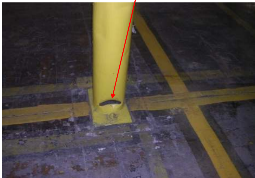
An example of a damaged column.
