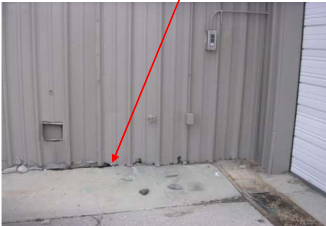
Left side rusting at bottom.
