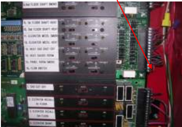
Bypassed input 16. Flow Switch.
