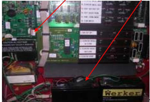
Disconnected from power and from backup battery.
