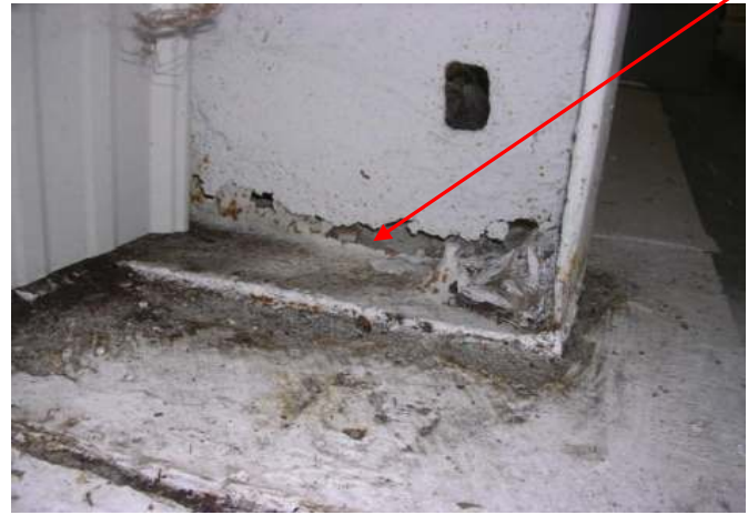
An example of a rusted through column at the bottom.
