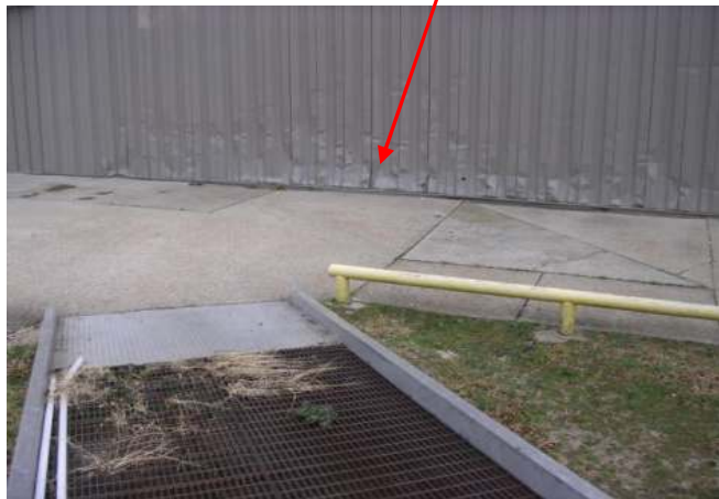
Left side near the inclined ramp damaged.
