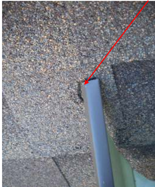
Shingles being cut by gutter on back porch. Gutter cutting shingles both ends on back porch.
